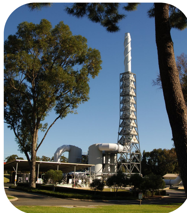
Figure 24: Subiaco WWTP odour control
