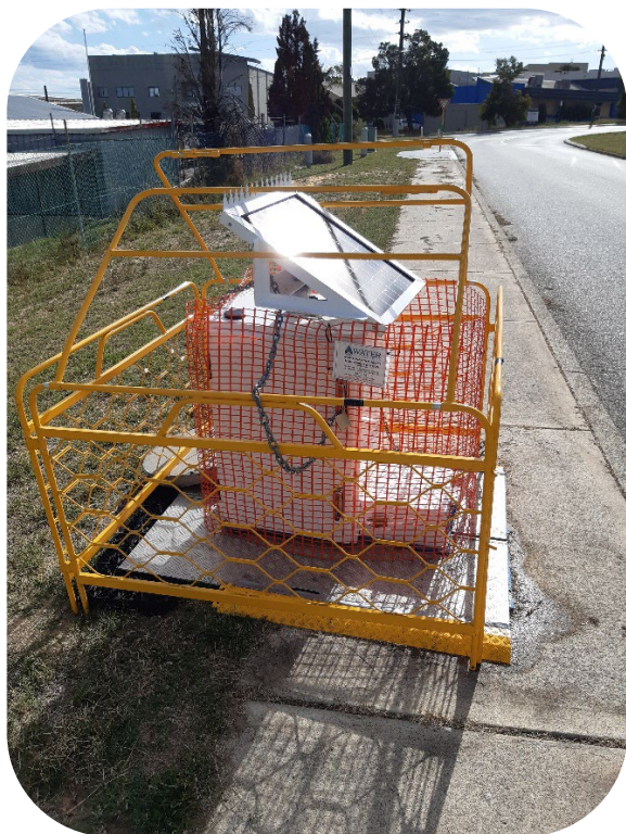
Figure 5: Portable sewer wastewater quality monitor
