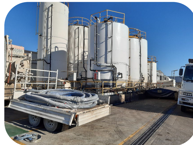
Figure 6: Receival and storage tanks at a waste treatment facility
