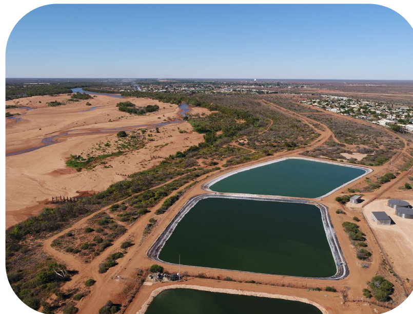
Figure 1: Carnarvon WWTP – wastewater treatment ponds
