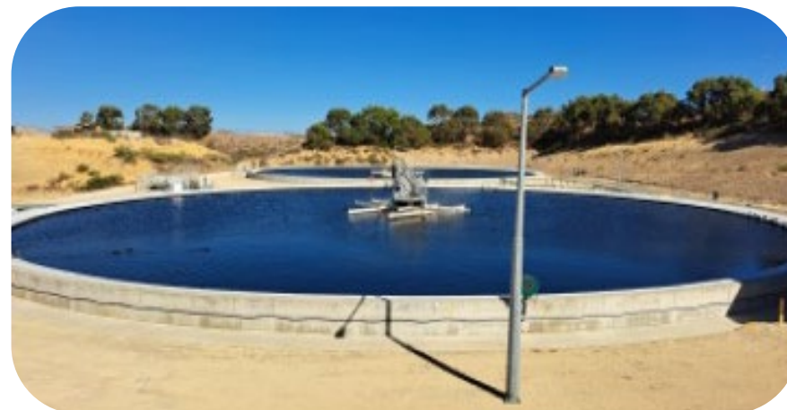
Figure 9: Alkimos WRRF secondary clarifiers
