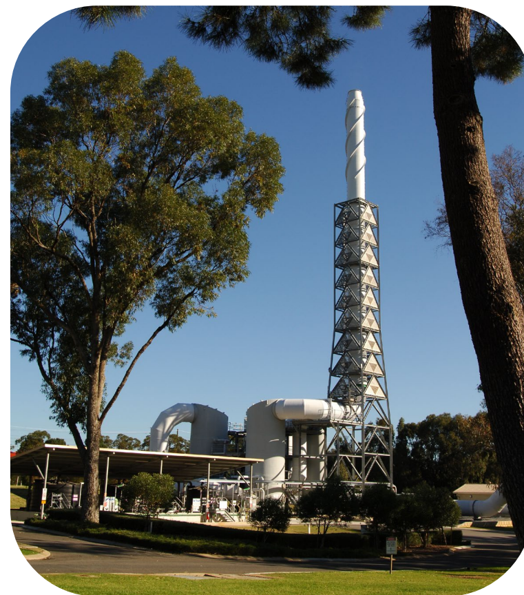
Figure 27: Subiaco WWTP odour control
