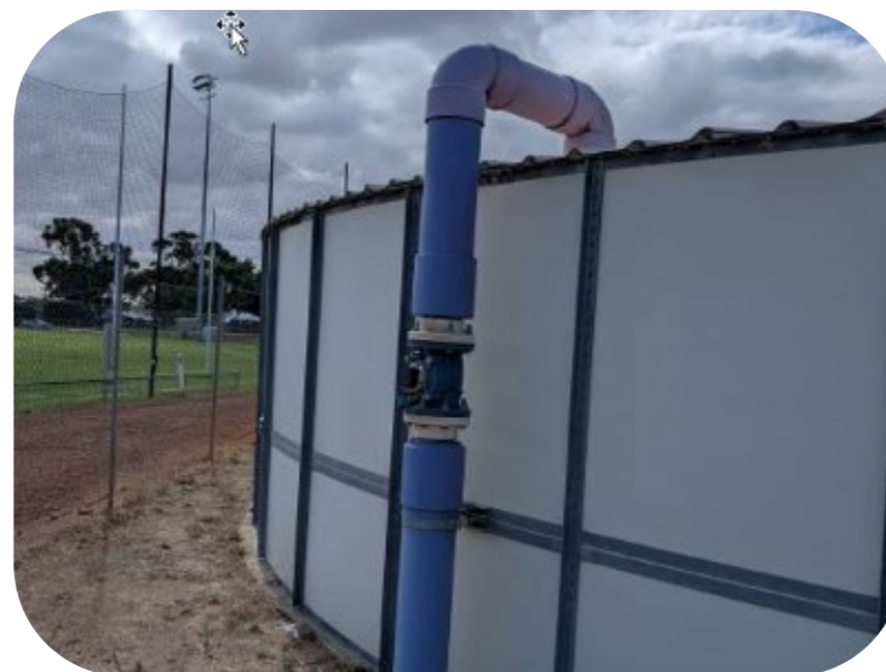
Figure 17: Auditing recycled water assets – Northam Harness Racing Club tank
