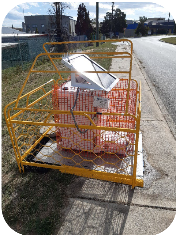
Figure 5: Portable sewer wastewater quality monitor
