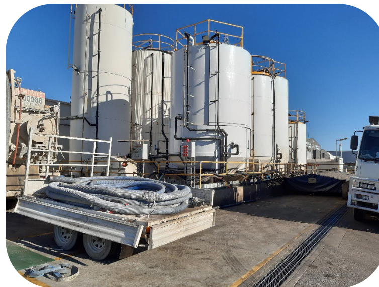
Figure 6: Reveal and storage tanks at a waste treatment facility
