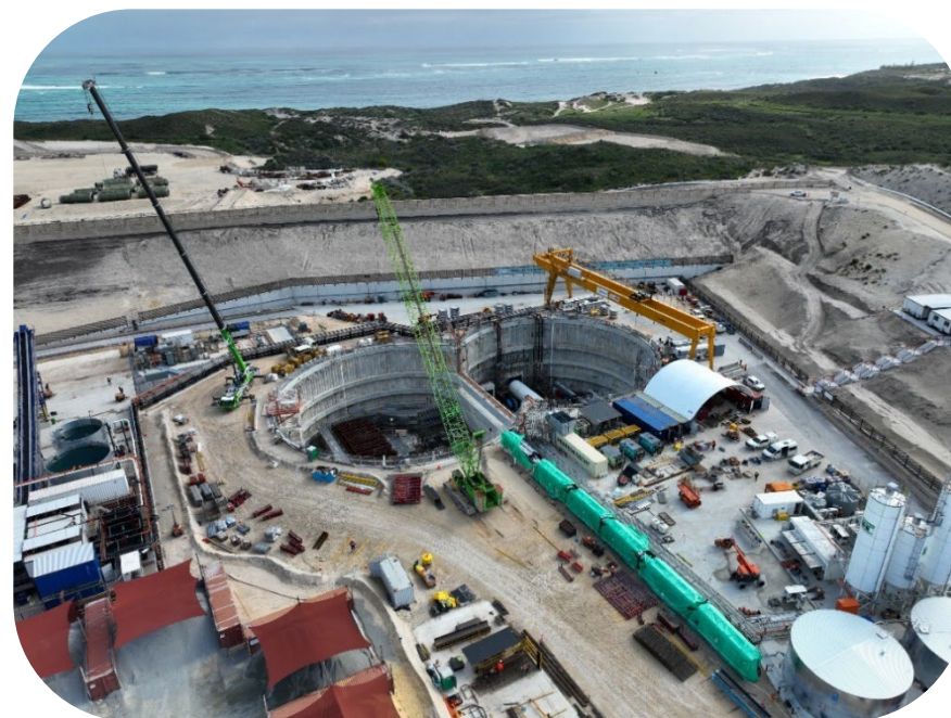
Figure 14: Alkimos seawater desalination plant - intake and outfall stations
