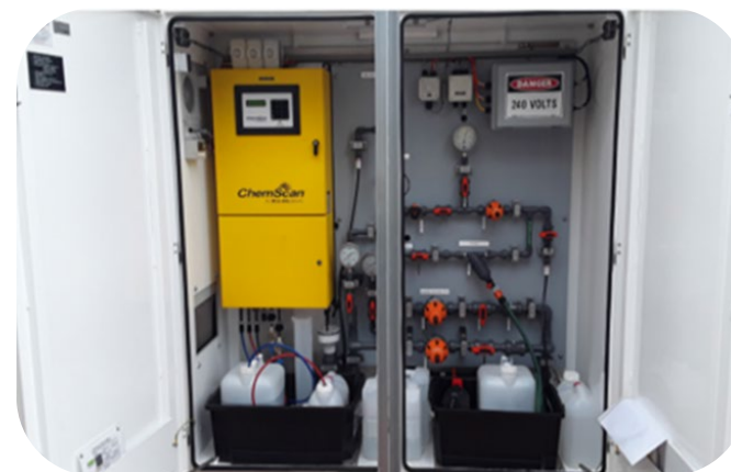
Figure 36: Advanced analyser installed on GAWS
