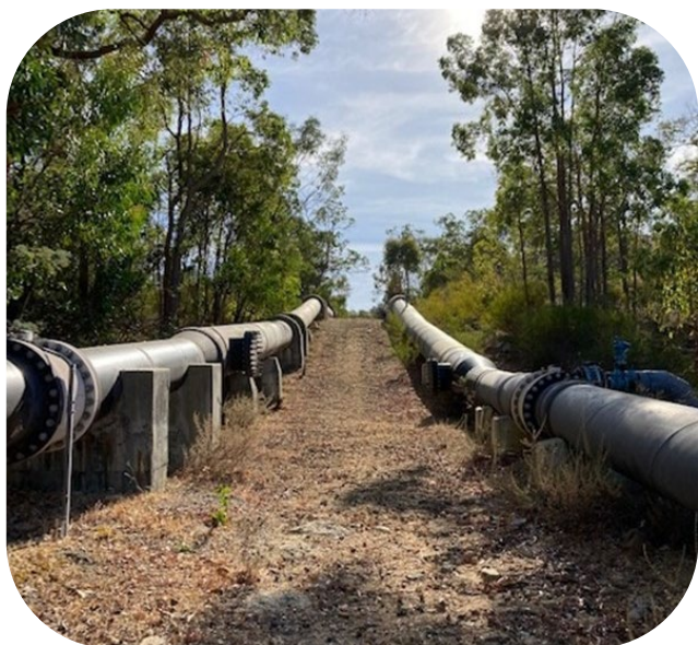
Figure 20: Dual Water Mains: Mundaring Weir to MWTP
