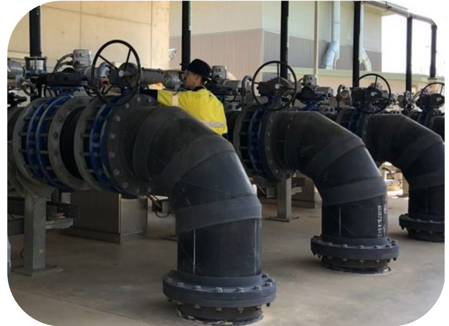
Figure 17: Mundaring Water Treatment Plant UV
