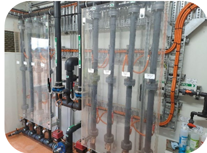
Figure 19: Horrocks WTP CEC cells – pretreatment bank
