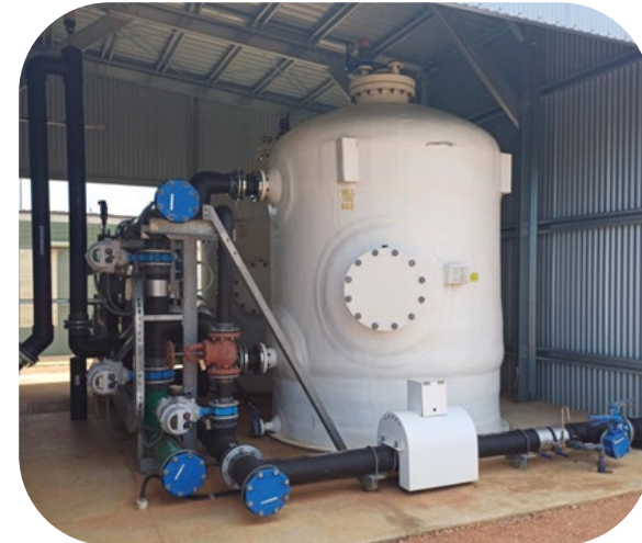
Figure 29: Granular activated carbon filters at Fitzroy Crossing
