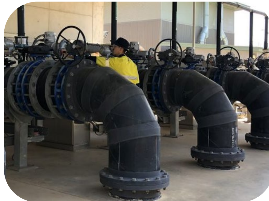
Figure 17: Mundaring Water Treatment Plant UV
