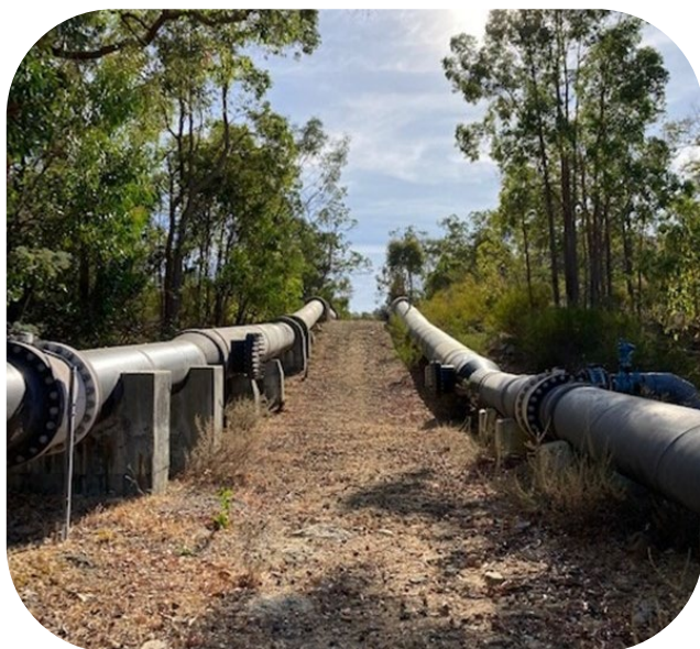
Figure 20: Dual Water Mains: Mundaring Weir to MWTP
