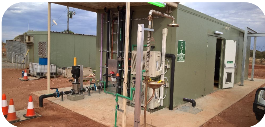
Figure 15: Wiluna EDR plant
