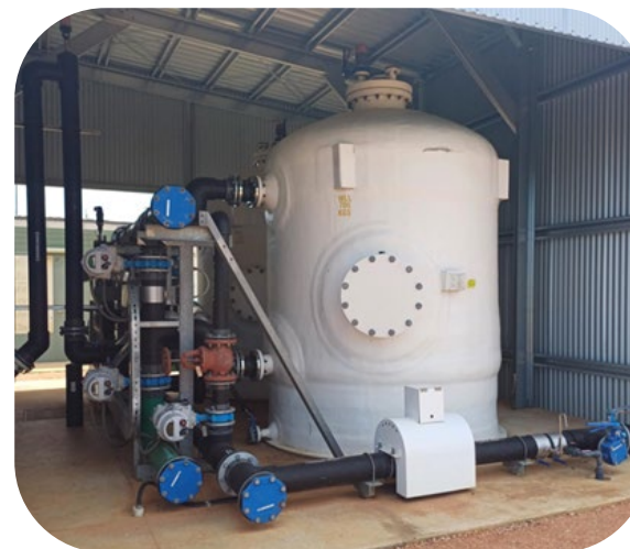
Figure 29: Granular activated carbon filters at Fitzroy Crossing
