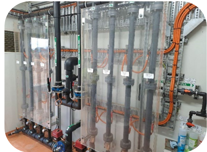
Figure 19: Horrocks WTP CEC cells – pretreatment bank
