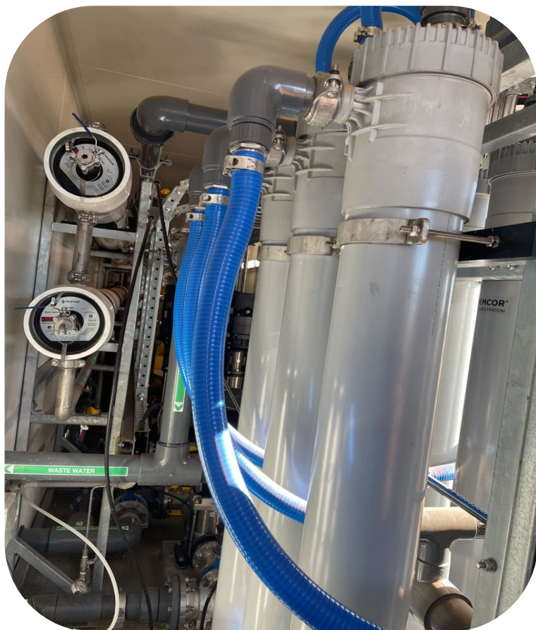
Figure 12: Kiwirrkurra ultra filtration and reverse osmosis treatment plant
