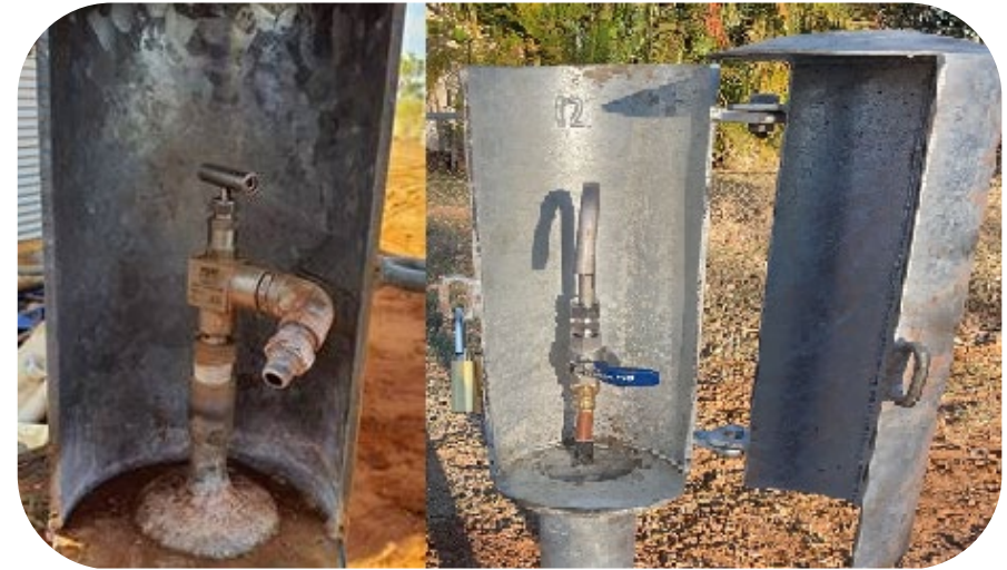
Figure 6: Older style tap (left) and newly installed sample tap
