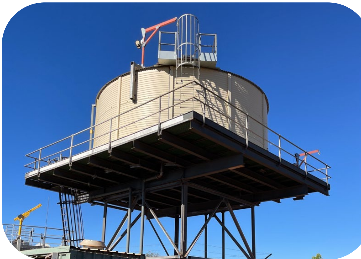
Figure 1: Wakathuni elevated tank
