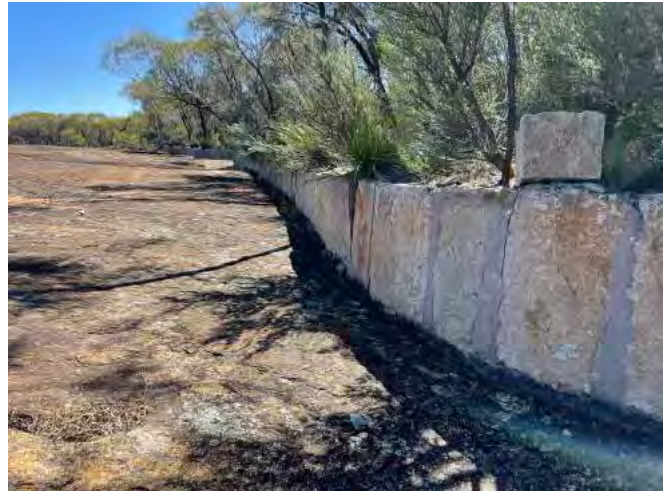
Karalee Rocks, diversion walls installed along edge of original gutter used by Aboriginal people.
