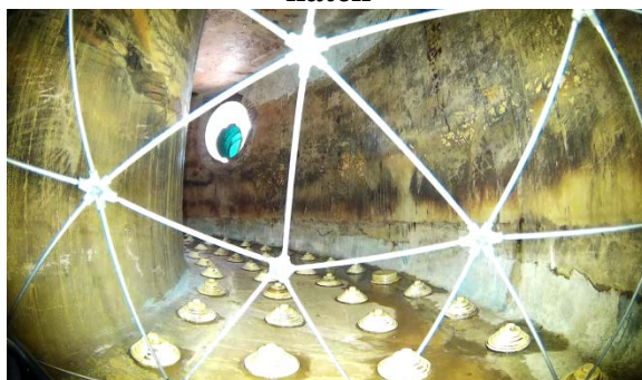
Photo 18 - Inside of an odor scrubber using a caged RPA
