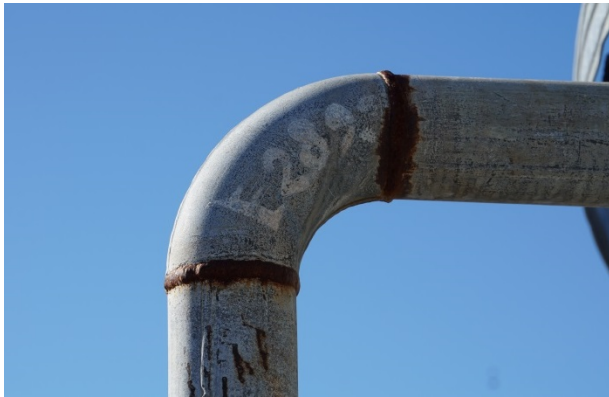
Photo 12 – Tank inlet pipe.
