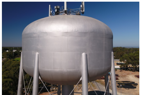
Photo 15 - Overview of satellite tank
