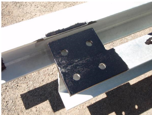
Photo 2 – Coating on galvanised cleats to prevent crevice/dissimilar metal corrosion.
