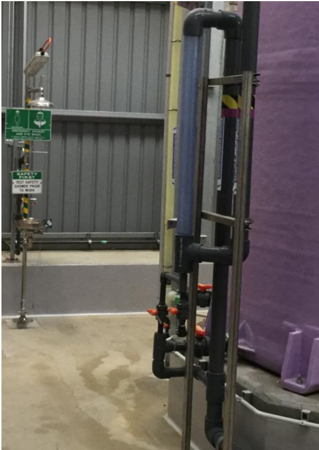
Figure 5-2: Overflow line with a transparent fillable seal pot visible from load-in panel
