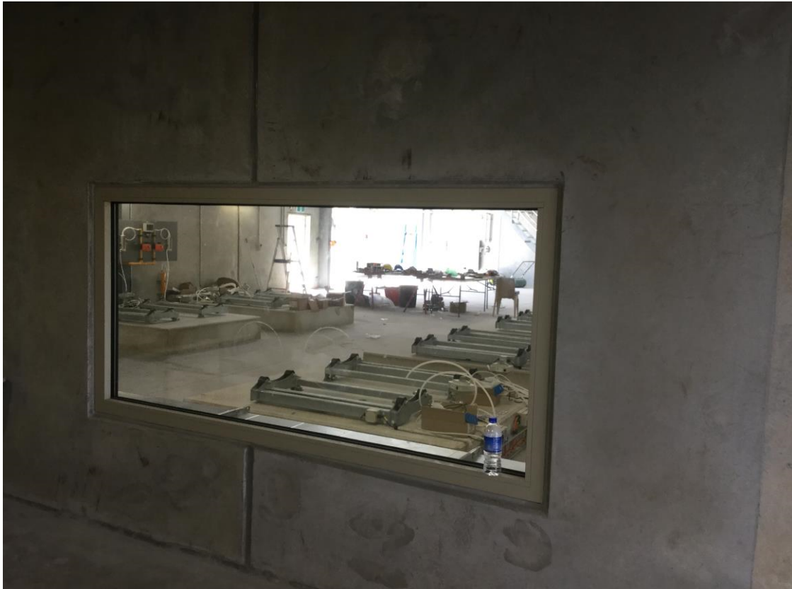
Figure 1: View of drum room from control/electrical switchroom
