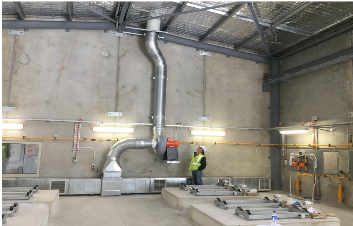
Figure 3: View of chlorine drum room ventilation (extraction) system
