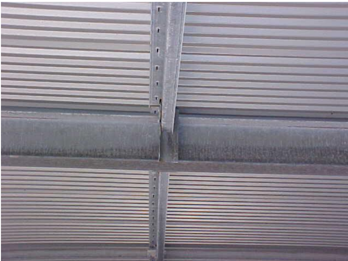
10. Corrosion of low grade “tek screws” (Minimum Class 4 required)
