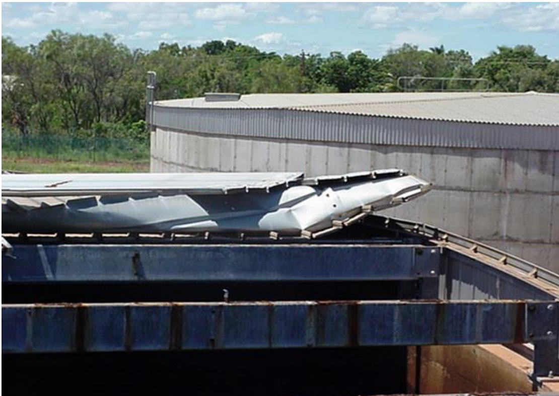
8. Corrosion of "Kliplok" sheeting system. Clips corroded due to lower coating class and crevice corrosion.
