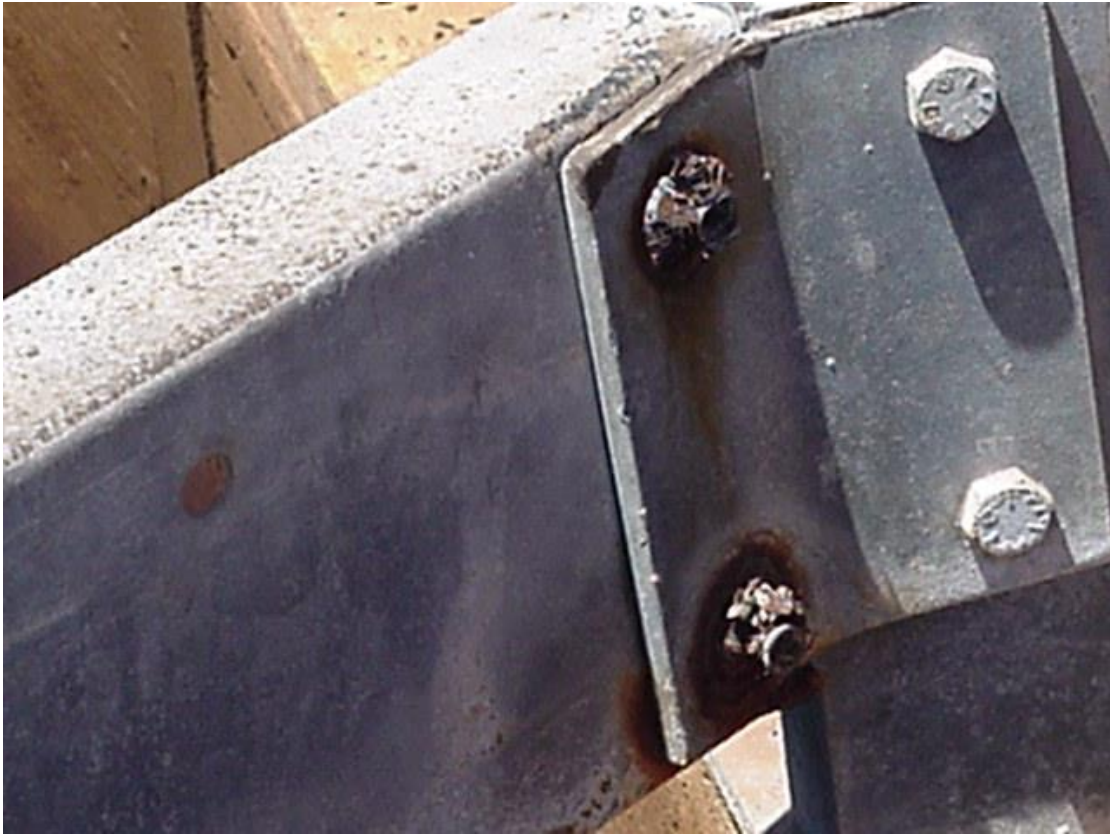
9. Corrosion due to absence of bituminous paint between interfaces
