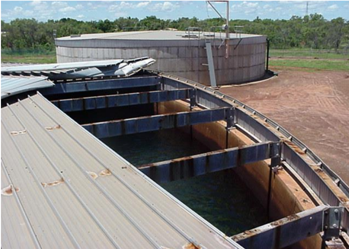
7. Roof sheet corrosion due to absence of bituminous paint between metal interfaces
