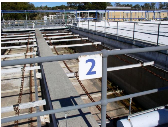
Photo 11 - Primary Sedimentation Tank in Wastewater Treatment Plant.
