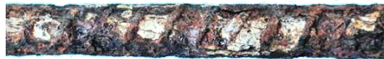
Photo 19 - Classification 3L. Majority of the surface covered with heavy dark brown rust.
