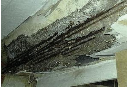
Photo 14 - Generalised chloride induced rebar corrosion. [Photo Courtesy: http://civil-engg-world.blogspot.com.au/2011/03/corrosion-induced-by-chloridesrcc.html ].
