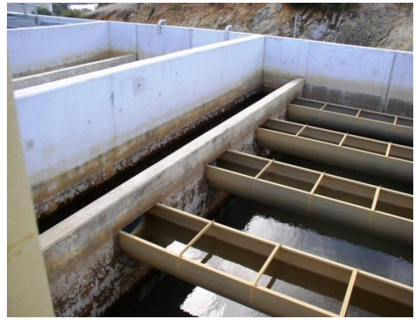
Photo 4 - Groundwater Treatment Gallery.
