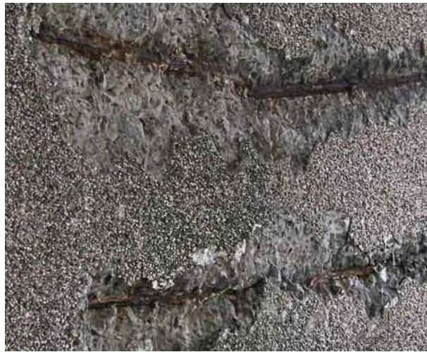
Photo 33 – Concrete failure due to Carbonation.
