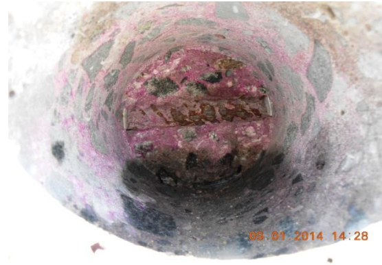
Photo 26 - Condition of concrete is alkaline (Refer: Pink colouration).
