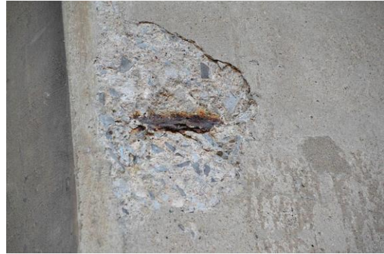
Photo 15 - Localised chloride induced rebar corrosion. [Photo Courtesy: http://www.en.wikipedia.org/wiki/Concrete_degradation ].
