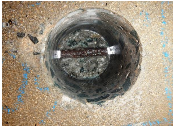
Photo 30 - Rebar condition (Rust Classification No. 2).
