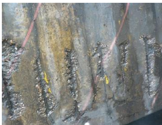
Photo 32 - Corrosion of the reinforcement due to chloride contamination.
