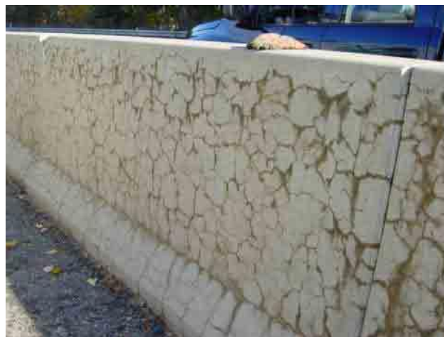
Photo 24 - Alkali-silica reaction affecting a concrete step barrier. [Photo courtesy: Federal Highway Administration, US Department of Transportation].
