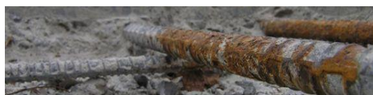
Photo 17 - Classification 2, Discrete blotches of corrosion products.
