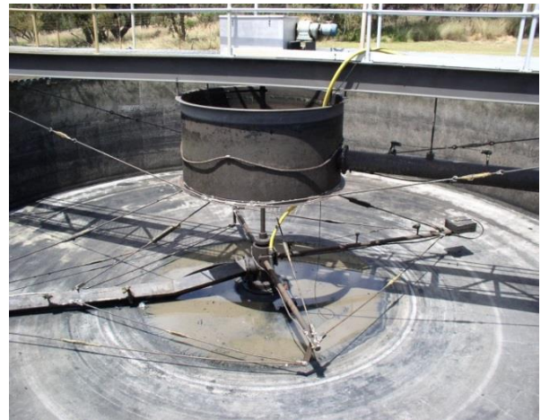
Photo 10 - Clarifier in Wastewater Treatment Plant.
