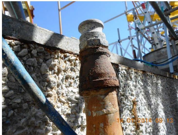
Photo 35 – Typical concrete surface attacked by Hydrogen Sulphide.
