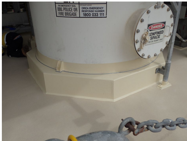
Figure 6 – Typical coating finish at the interface between concrete plinth and tank wall
