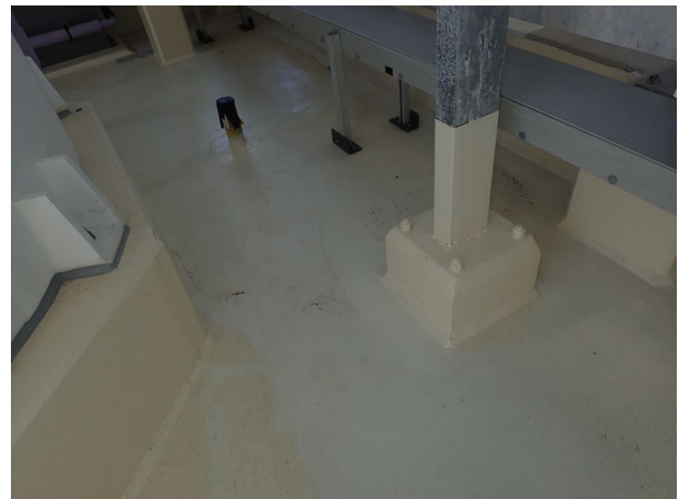
Figure 7 – Typical coating finish at the interface between concrete plinth and pipe supports
