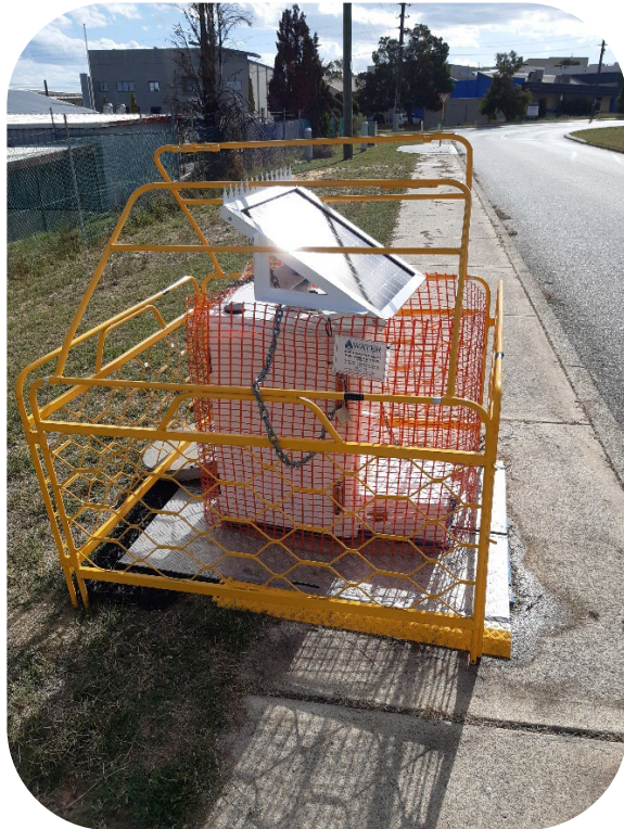
Figure 5: Portable sewer wastewater quality monitor
