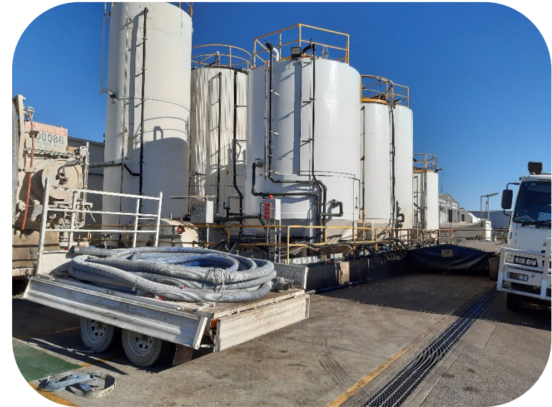
Figure 6: Receive and storage tanks at a waste treatment facility
