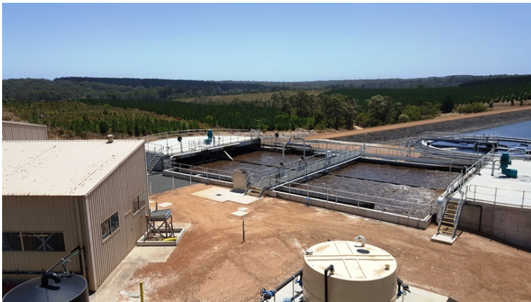
Figure 8: Margaret River WWTP – New oxidation ditch
