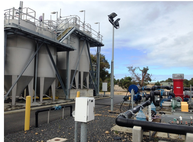
Figure 9: Kemerton WWTP – denitrification filtration system
