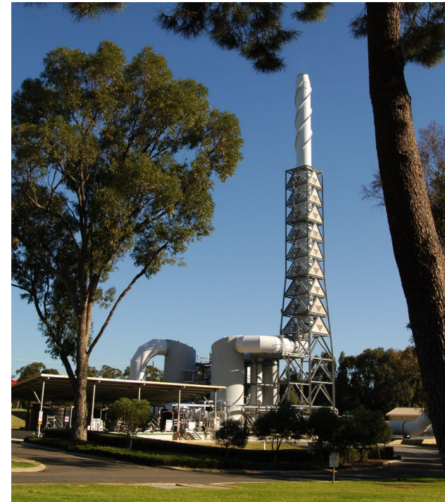
Figure 19: Subiaco WWTP odour control
