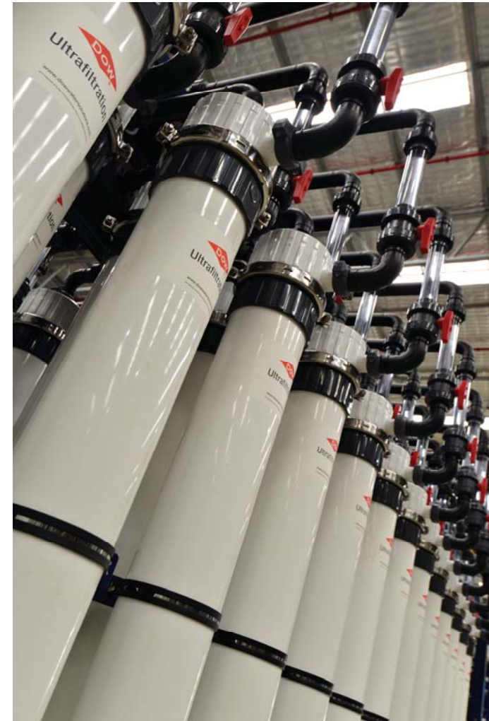
Advanced Water Recycling Plant
