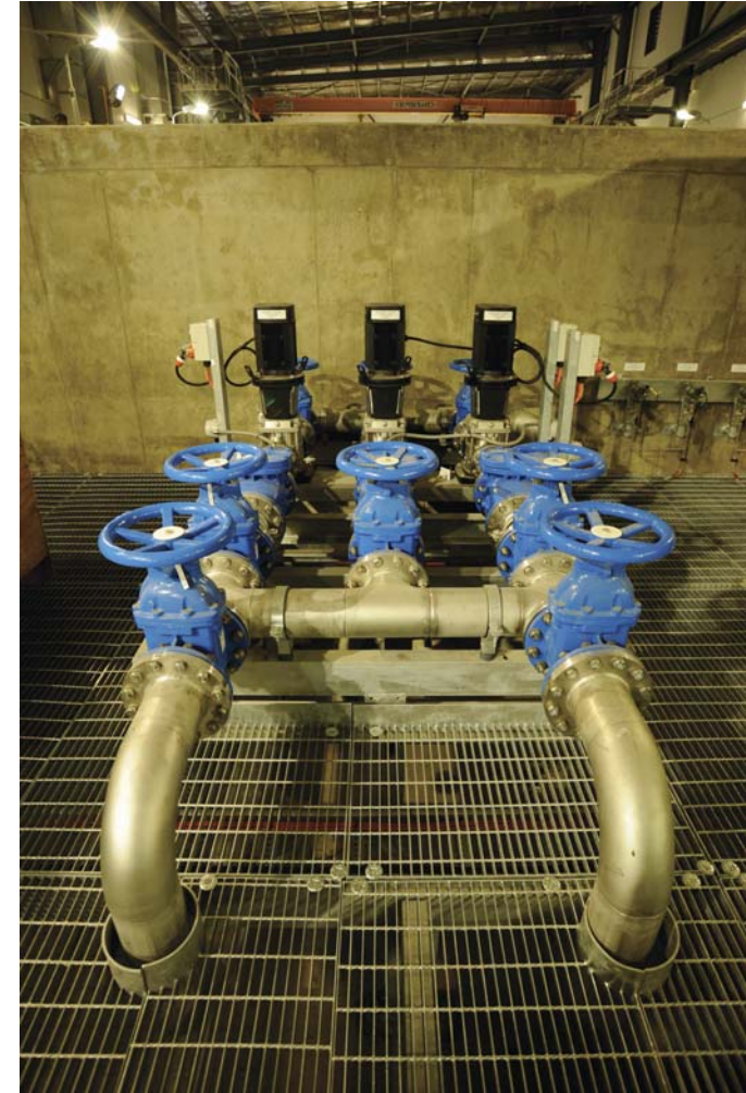
Valves inside Ravenswood Pumping Station
