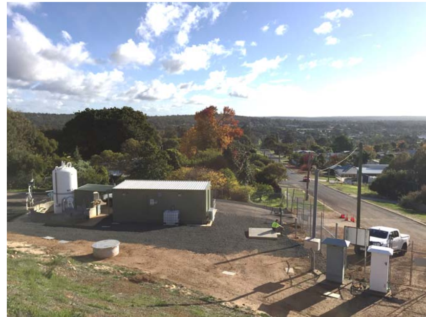
Electro-chlorination water treatment system at Horrocks
