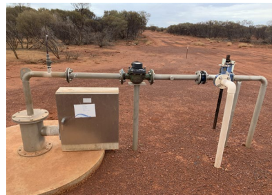
Sealed tanks and bores
