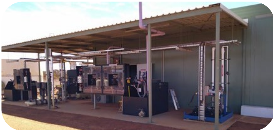
Figure 16: Mt Magnet EDR plant – feed pump and chemical dosing
