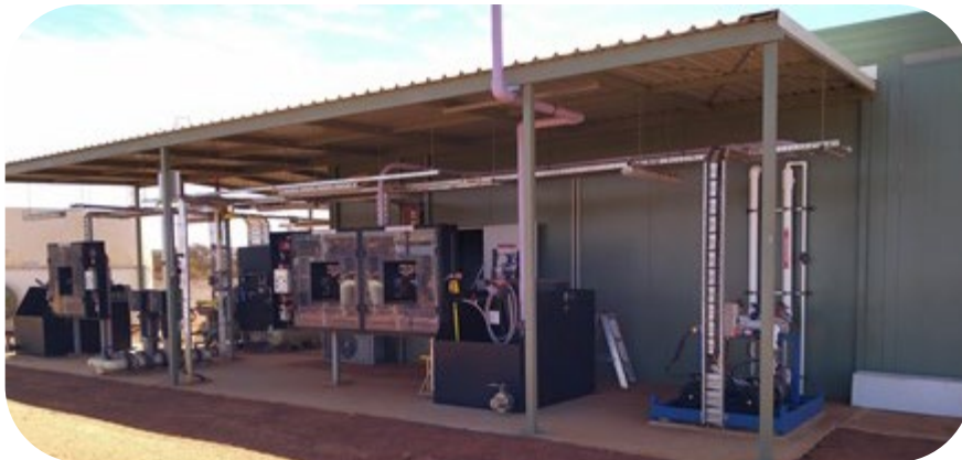
Figure 18: Mt Magnet EDR plant – feed pump and chemical dosing
