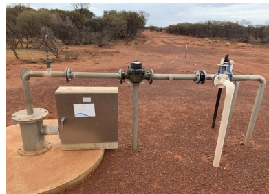
Sealed tanks and bores
