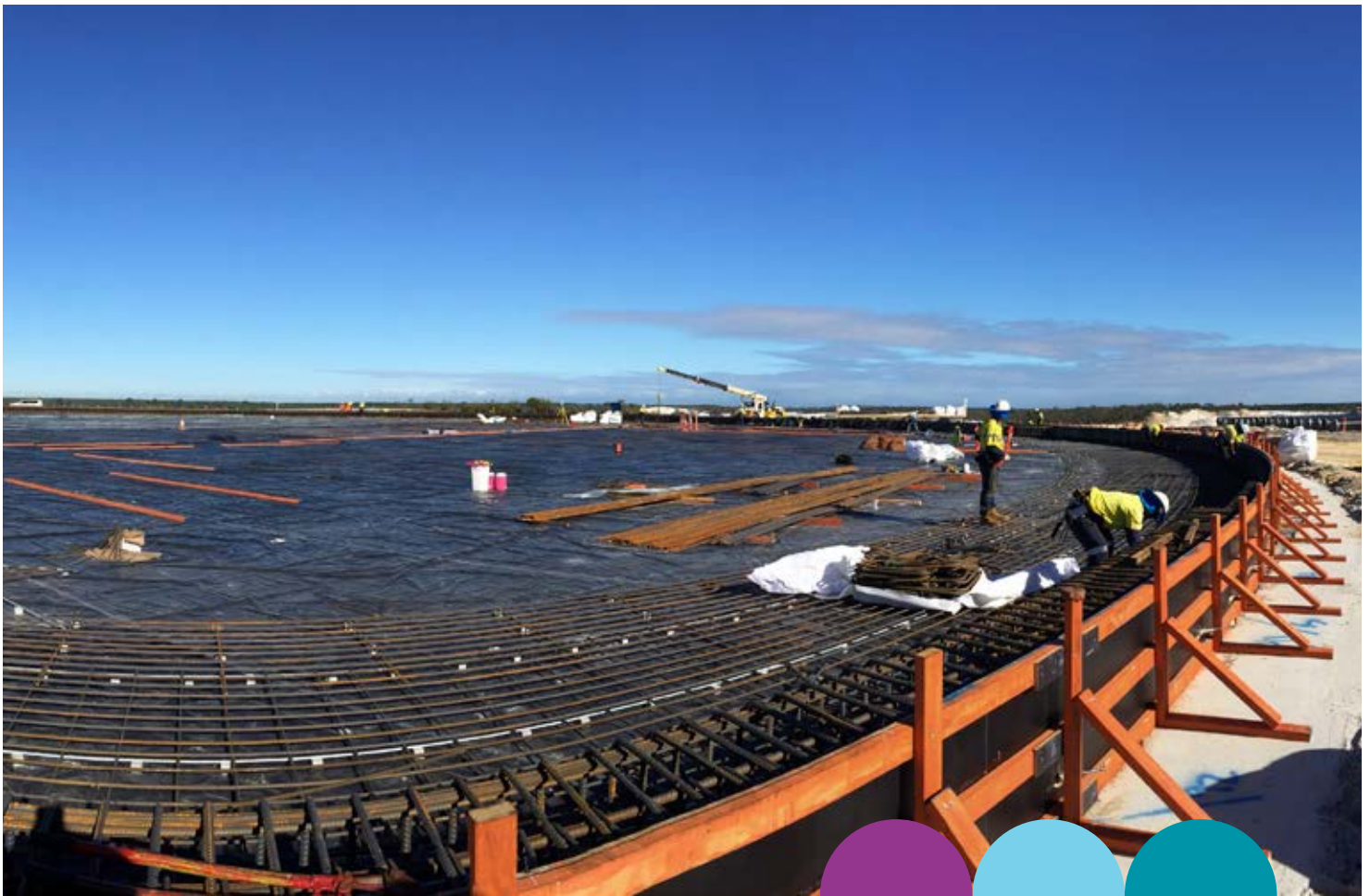
Construction of the Ellenbrook water storage tank will create more than 200 jobs during construction phase.
